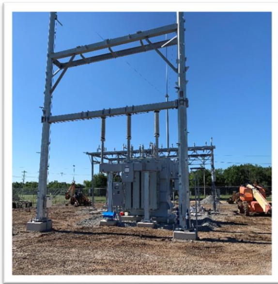
Looking to the North Harmony Substation
