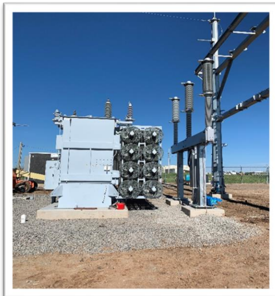
Looking to the East at the North Harmony Substation
